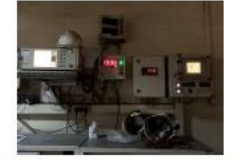
Figure 8: Electric Arc Furnace Temperature Control
